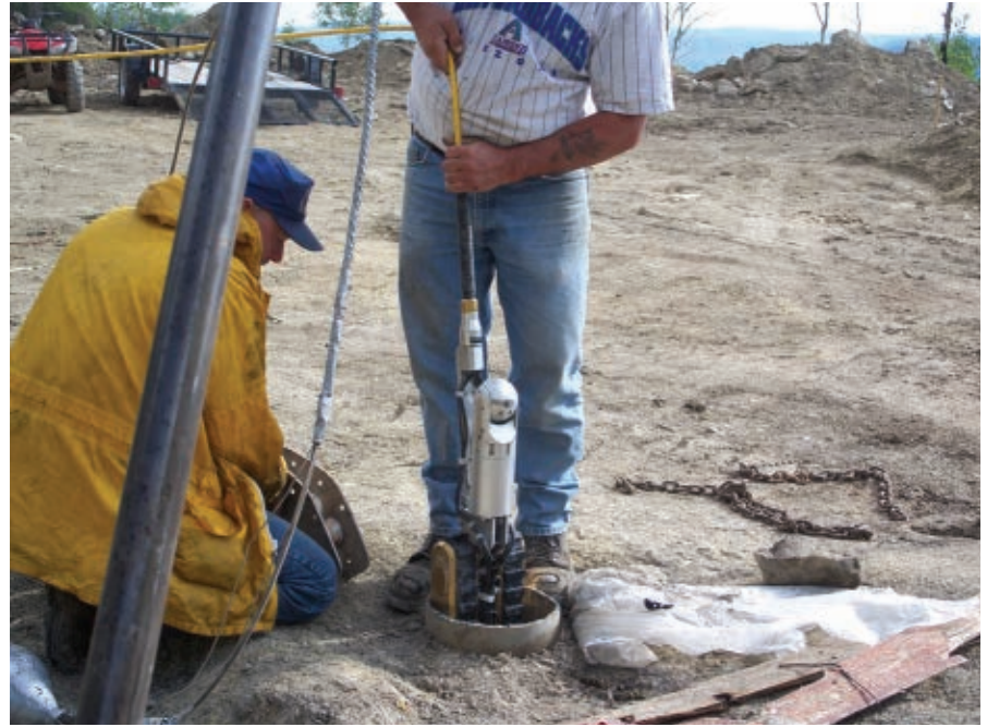
A camera robot being inserted in a bore hole at Crandall Canyon Mine in Utah.
