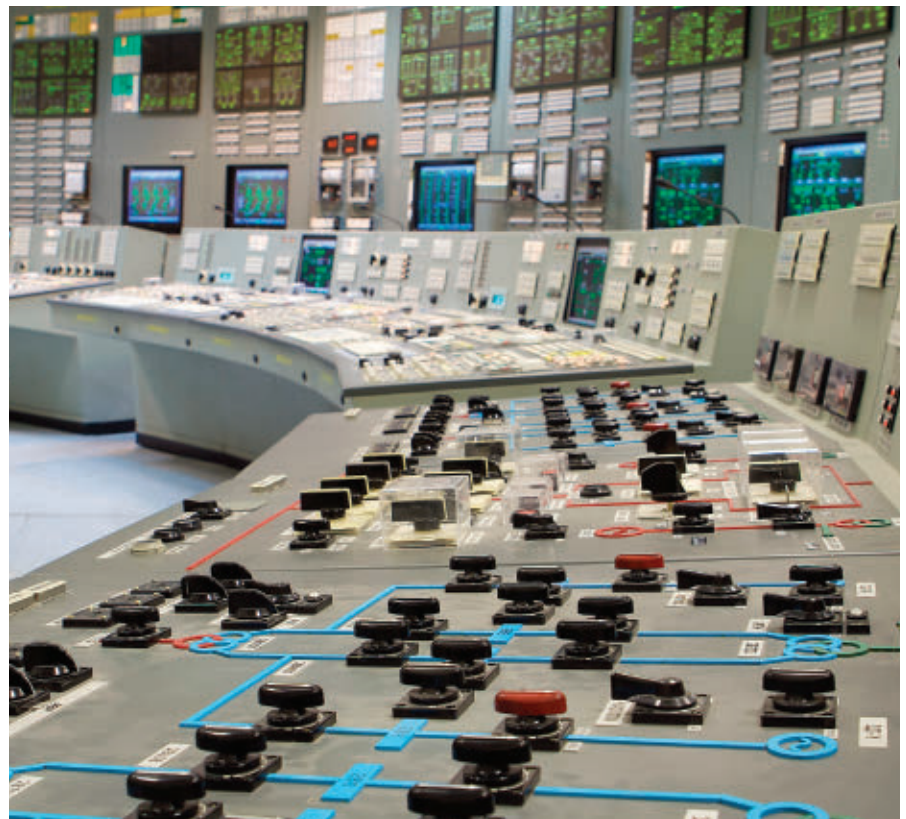
Control room of a nuclear power plant.
