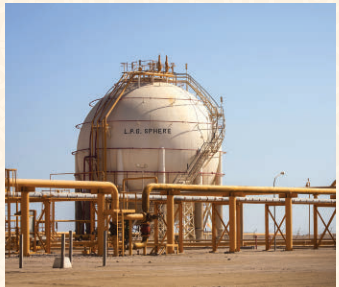
An oil and gas processing plant in Egypt.
